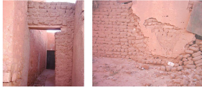
Fig. 1. A typical example of decrepitude of an adobe wall. Source: 3rd year students of architecture department (2005–2006).
