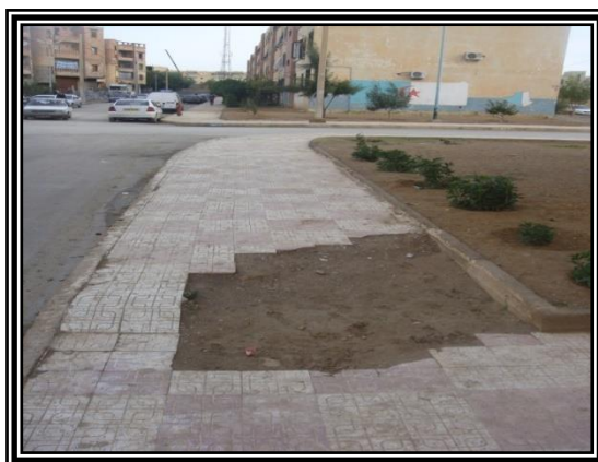
Photo No. (07): shows the deterioration of the sidewalks and the lack of maintenance.
