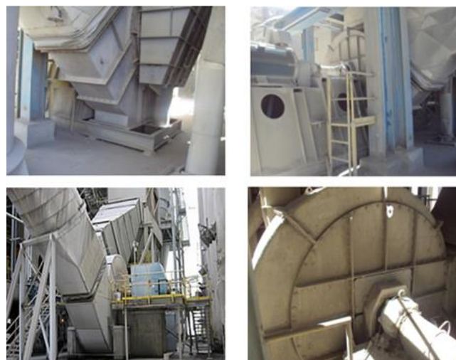
Figure 1. Images of cement draft fan.
