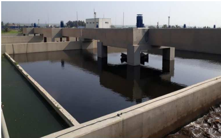
Fig.1 The sewage aeration tank of El-Kerma wastewater treatment plant in Algeria
