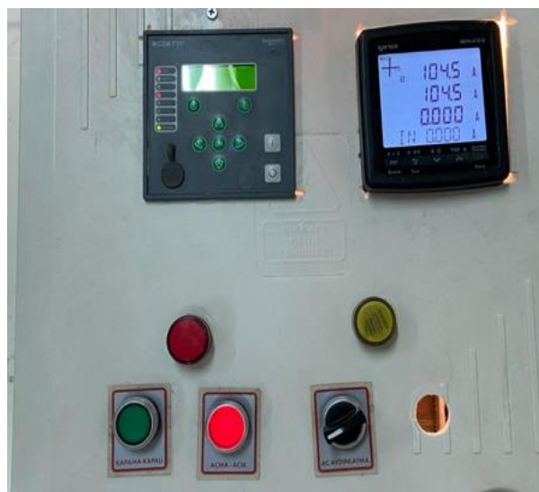
Fig. 10 MICOM P111 Overcurrent Fault Status After Applied Scenario
